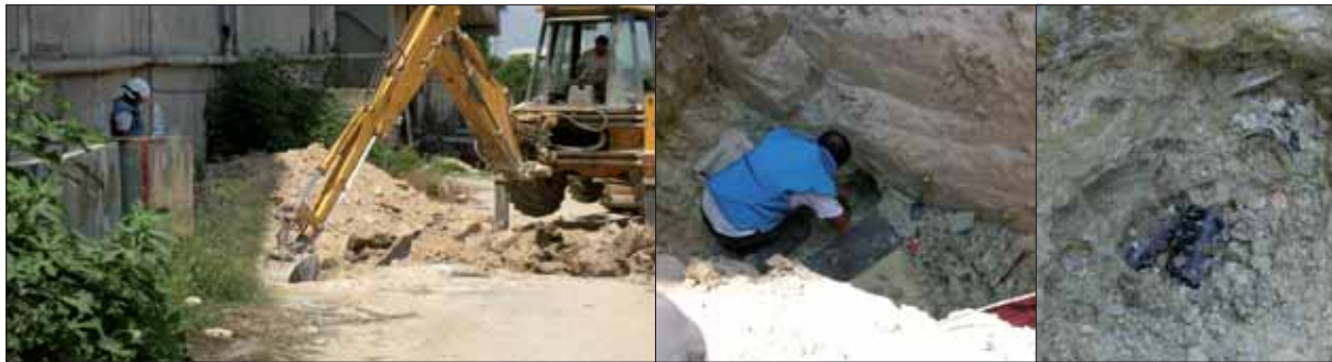
Figures 7-9: On 26 June 2007 Swedish Rescue Services Agency (SRSA) were called to a site in Deir Qanoun Al Nahr to investigate a complete failure of a 155 mm cargo projectile. The projectile's entry hole was just by the back wall of a block of flats. Upon arrival, they found three M85 duds in the middle of the road between the block of flats and an orange grove. The entry hole was excavated and M85 bomblets were found at various depths along the entire entry hole, but most of them just before the projectile casing, which was a CL3013-E1. No bomblets remained inside the projectile. Photos: Robert Ericsson/SRSA
